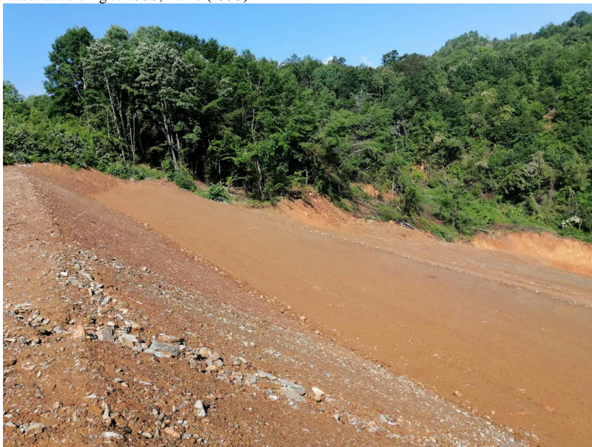
Figure 1. Section of highway E-75, Corridor 10, Gornje polje-Caričina dolina, Cut V, Level II
